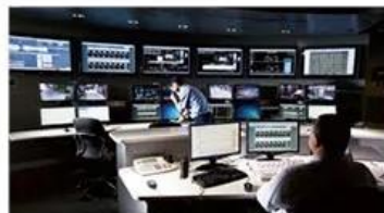
Command and control center
